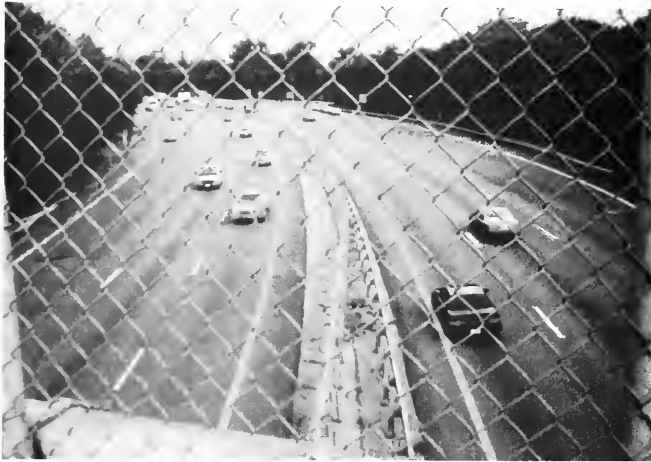
B -- Looking west from Grant Avenue overpass at strong post block-out guardrail
